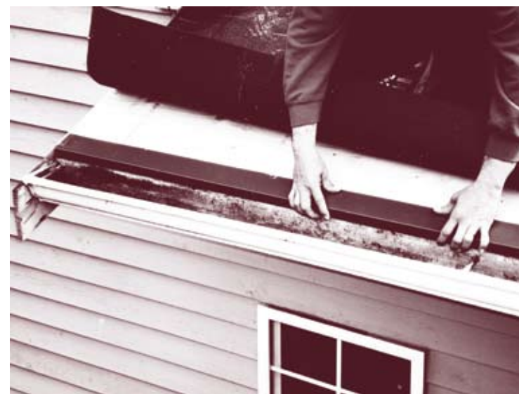
A corrosion resistant enamel coated metal strip is added to protect the bottom edge of the plywood sheathing.
