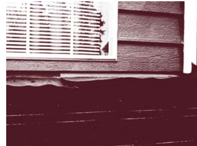
Old roof-to-wall flashings.
